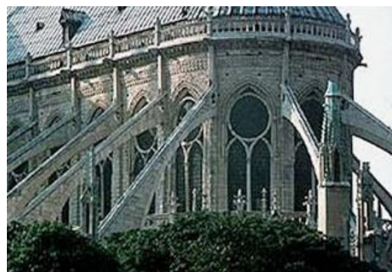
Fig 10. External buttress strengthening [3, 11].
